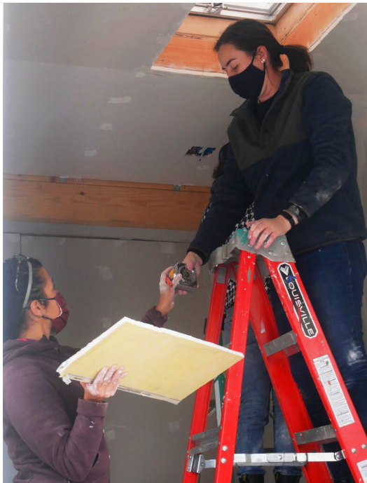
Jessica Earle, left, and Sarah Nelsen work inside a 100-square-foot tiny home in East Oakland, California, as part of a Dykes With Drills workshop on Jan. 3, 2021. (Photo by Katie Lauer)
